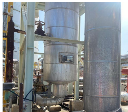
Gbr. 1 Ammonia heater (Ea-2001)
