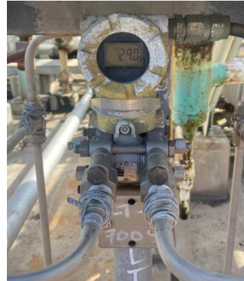
Gbr 5. Level transmitter (LT-7005)
