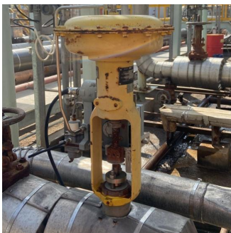
Gbr. 4 Control valve (LV-7005)
