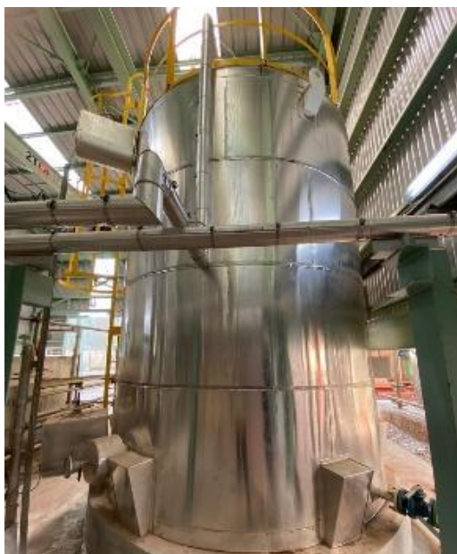
Gbr. 1 Coating Oil Tank
