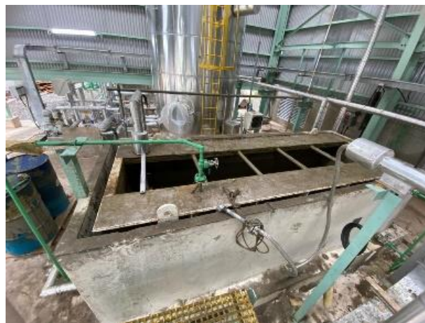
Gbr. 2 Coating Oil Heater Tank
